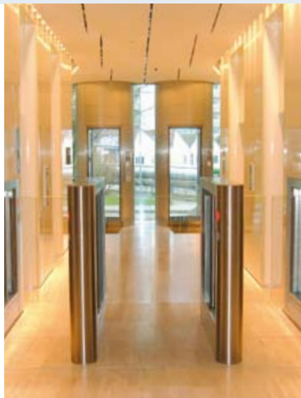
Double access control - sensor barrier with extension unit and Orthos personal interlock system in the background
